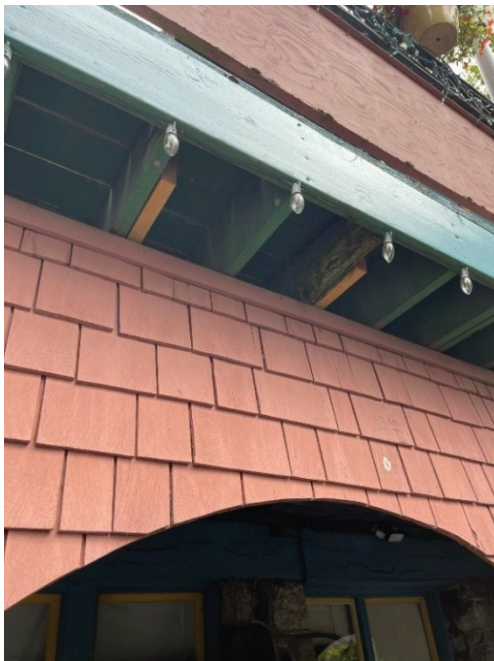
Figure 5: Deck Joist Rot
